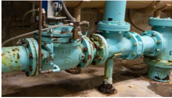
Aging Water Infrastructure
